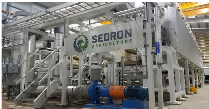
Figure 1. SEDRON Evaporation System.
