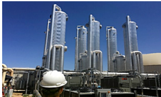
Figure 6. Biogas cleaning and upgrading system.
