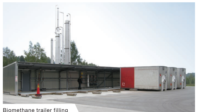
Biomethane trailer filling
